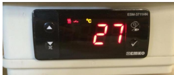
Figure 4. Temperature controller ON.
